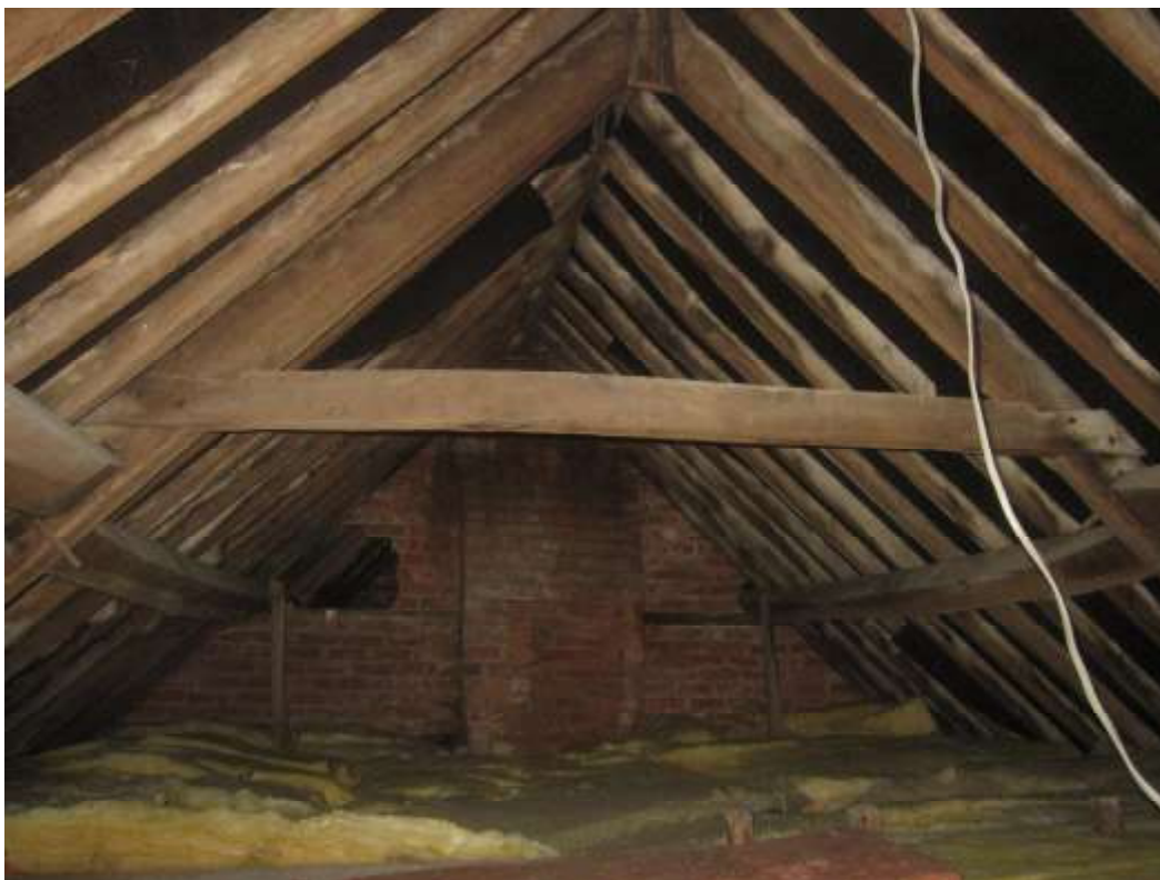
Roof structure to house: central room looking north, with lapped and nailed collar
