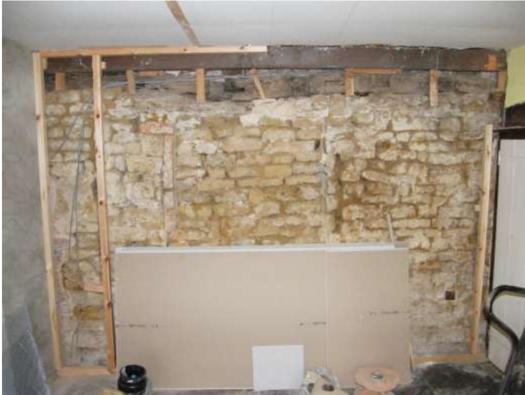
Rear east wall of No 1, with timber plate on top of stone ground floor wall
