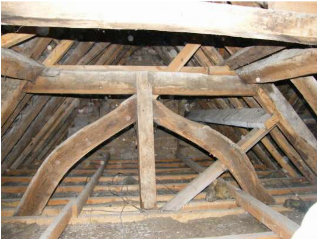
South face of Truss T1 with decorative bracing between tie-beam and collar
