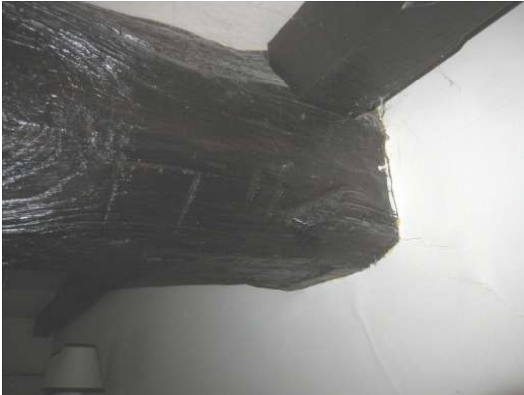
Pyramid chamfer stop of early type to ceiling beam of central room
