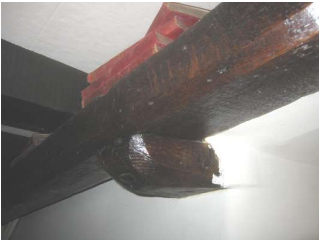
Oak plate on corbels, supporting ceiling joists to east side of central room
